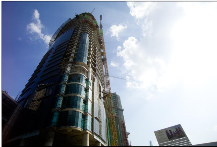
Figure 1: A construction site of high rise commercial building located near MidValley, Kuala Lumpur, Malaysia.
